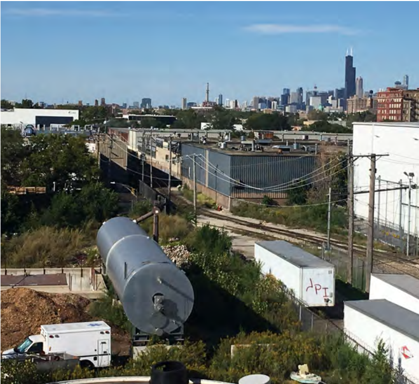
Full-scale anaerobic digester at The Plant.
